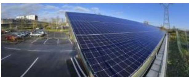
Figure 23 – Ombrière photovoltaïque de Lomme (France).
